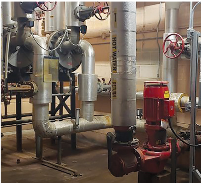
This hydronic heat distribution system was retrofitted at CFB Kingston to decrease energy consumption and fossil fuel dependence, as part of the IDEaS Green Heat challenge.
