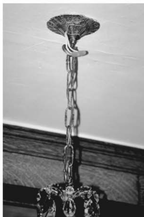
Figure 4. Exposed wiring on this lighting fixture does not meet electrical codes.
