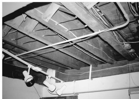
Figure 1. An example of unprotected basement ceiling joists.
