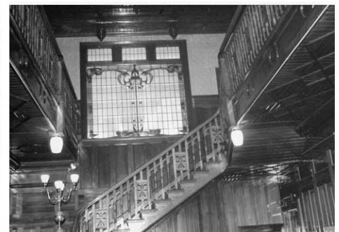
Figure 2. Open staircases allow fire and smoke to spread quickly.
