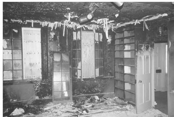
Figure 4. The Second Generation Room of Billings Estate Museum was extensively damaged by fire.
