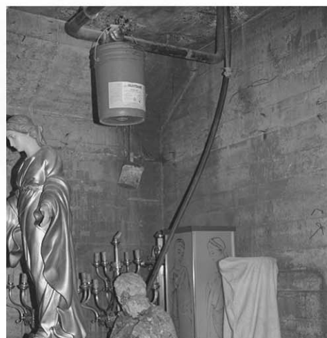
Figure 4. Water leak from plumbing pipe.
