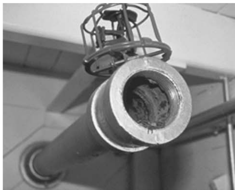
Figure 1. Sediment in dry-pipe system. Note the wire cage protecting the sprinkler above the pipe.
