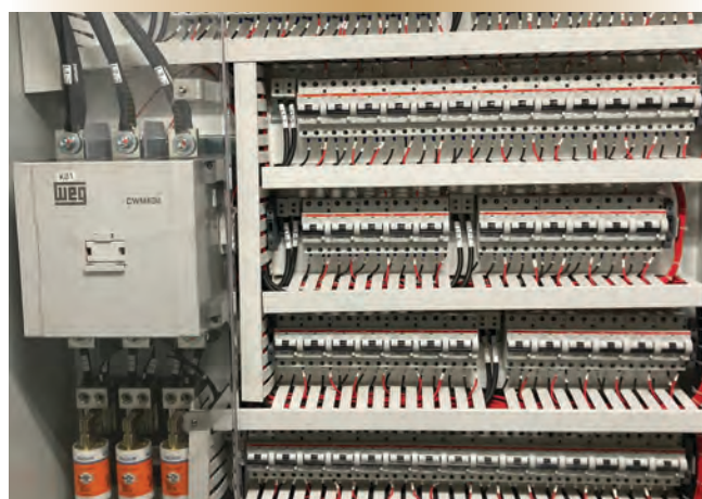
Figure 3. De-icing heating panel showing breakers.
