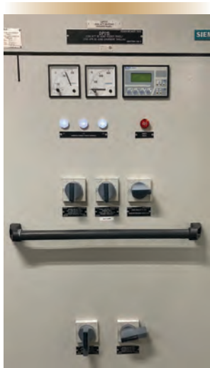
Figure 2. Main 220-V aft de-icing feeder panel.
