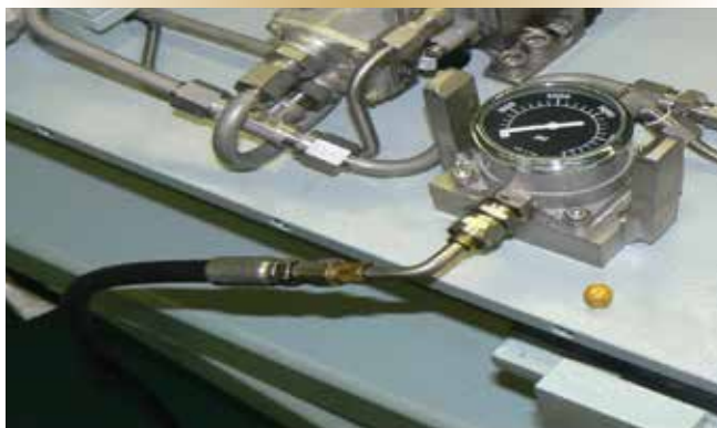
Figure 6. Pressure Gauge to be Monitored
