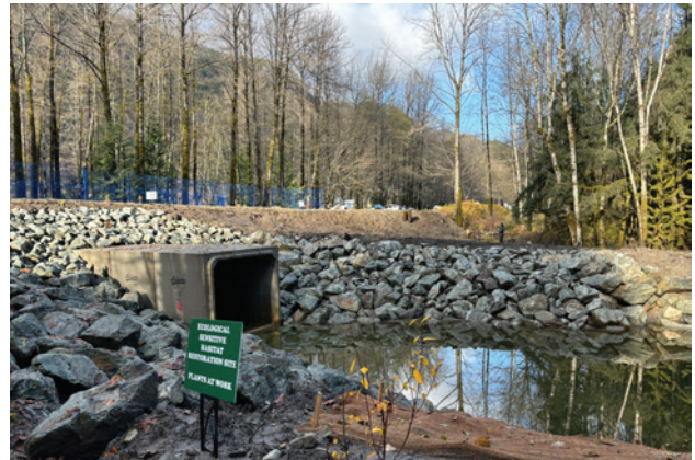
Box culvert upgrades restore natural coastal tidal exchange between the river, estuary and ocean even at low tide or during periods of low flow. (Photo by Sydney Bryce, DFO)
