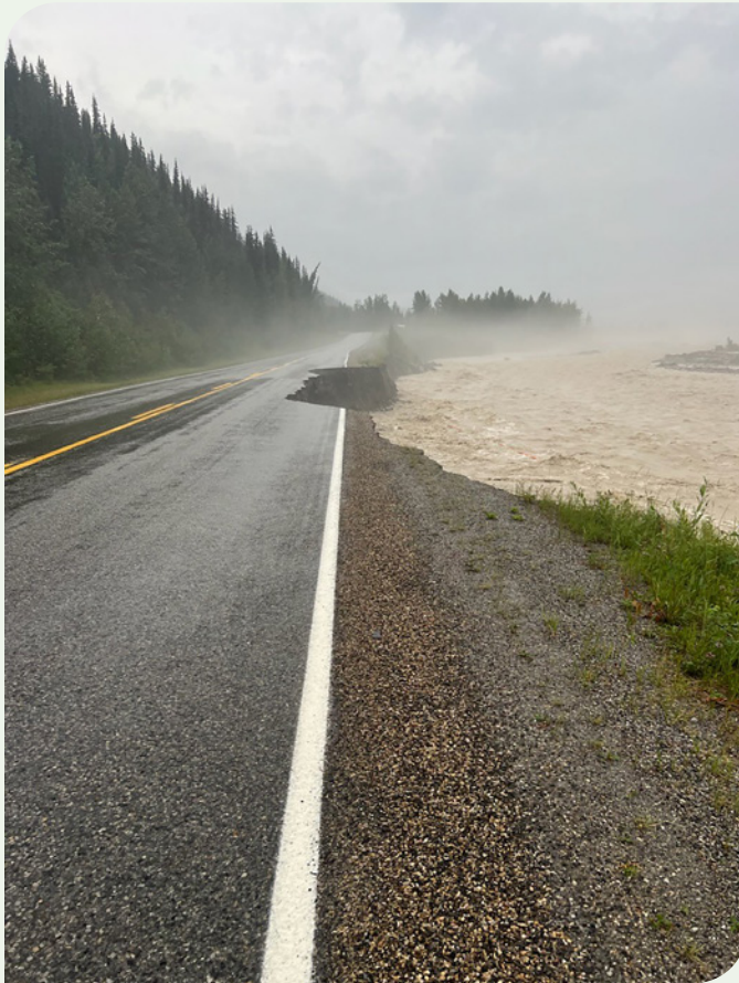
Washout section of the Alaska Highway in summer 2024.
