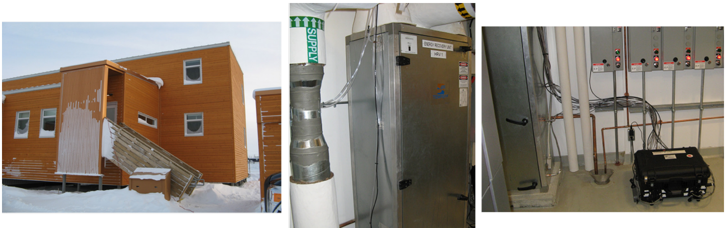
Figure 4: Triplex on CHARS Campus and deployed dual core unit and dedicated data logging system.
