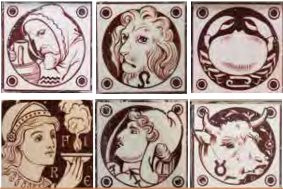
Tiles along the ceiling feature astrological signs that were found during rehabilitation. They were not on any drawings or plans and were revealed after four layers of lead paint were removed. For an unknown reason, Sagittarius is missing.
